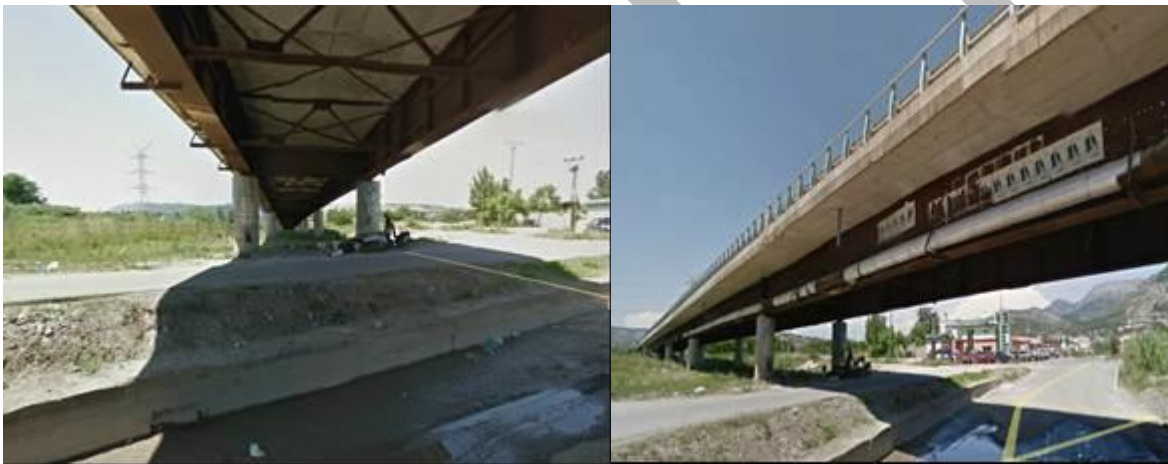
Figure 3-33 Existing bridge over Drini river in Lezhe (225m long) - View of the piers, steel girders and reinforced concrete deck
