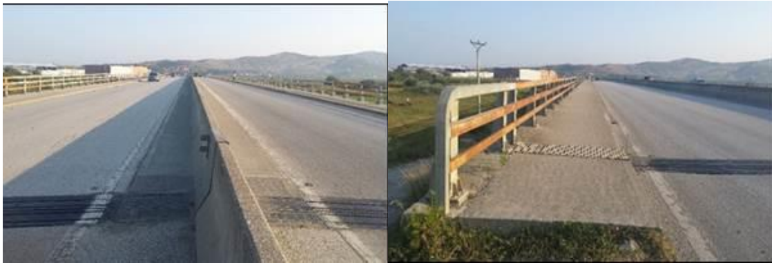
Figure 3-36 Existing bridge over Shkumbini river (300 m long) – View of the bridge platform and sidewalk
