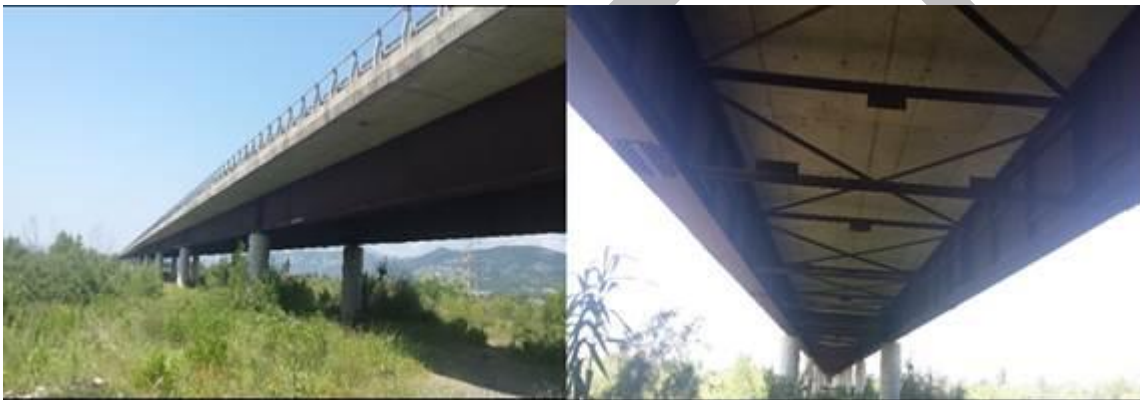
Figure 3-35 Existing bridge over Mati river - view of the piers, steel girders and reinforced concrete deck
